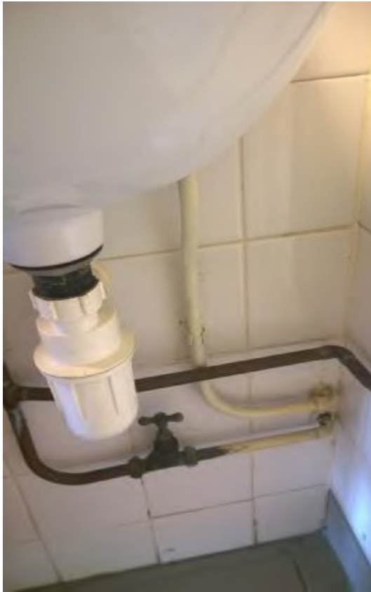
Isolation valve in kitchen area
